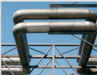
Pipelines subject to pressure
